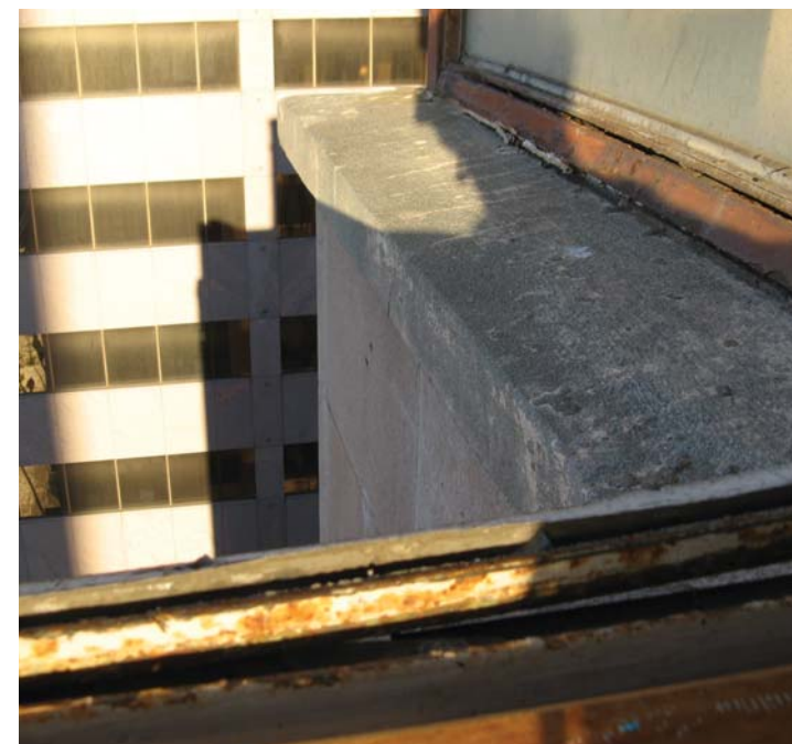
Typical tenth floor window exhibiting deterioration
