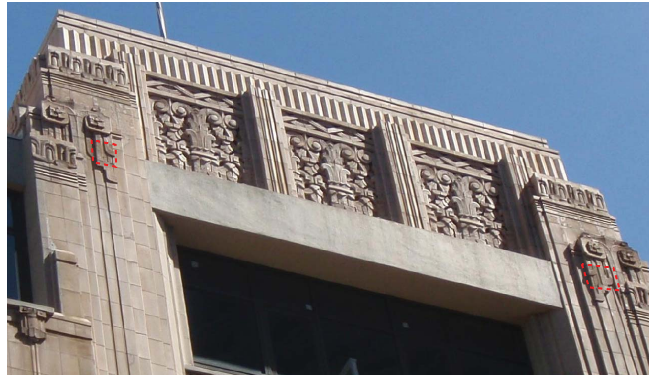
Terra cotta (shown in dashed rectangle) is to be removed and salvaged to allow for the installation of window washing equipment
