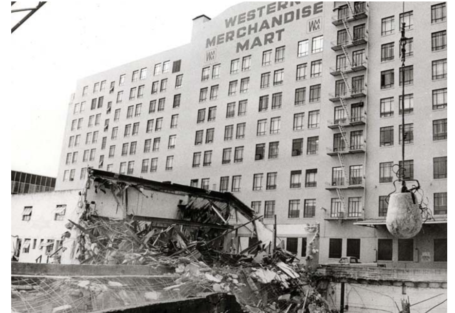
Demolition in preparation for Mart 2 construction with view of Stevenson Street facade, 1973 (Market Square Archives)
