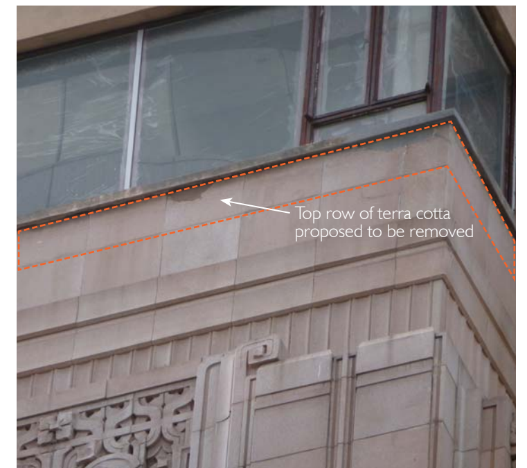
View of tenth floor windows and terra cotta proposed to be removed
