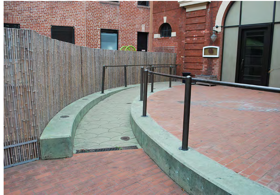
Inappropriate - paving materials should be in keeping with the character of Ghirardelli Square.
