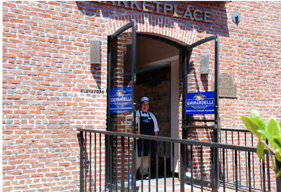
These steel replacement doors are compatible with the industrial character of the Woolen Mill and are therefore appropriate
