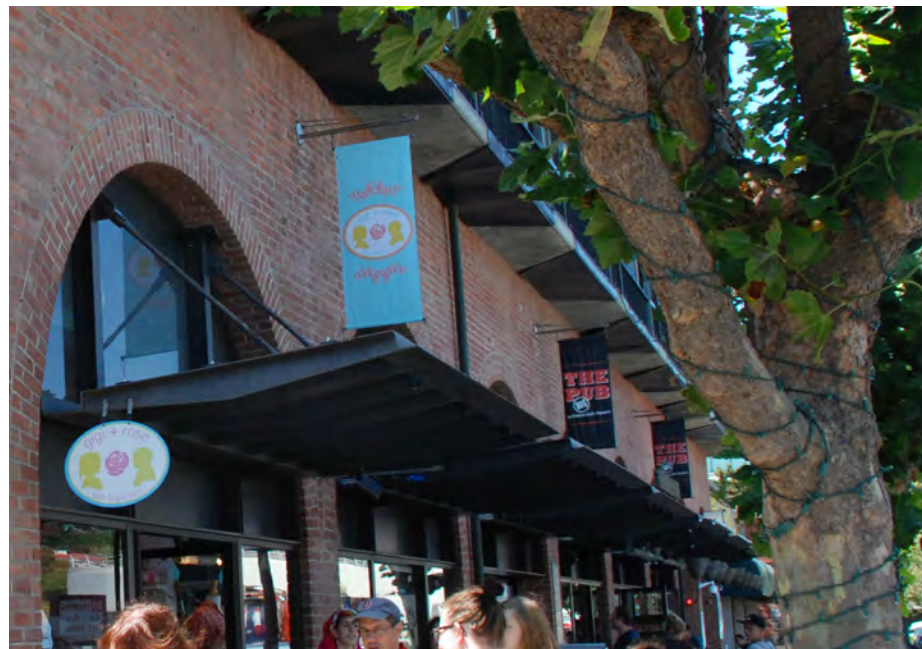
The tenant signs at the north facade of the Wurster Building include blade signs above the canopies that display contemporary designs that are acceptable.
