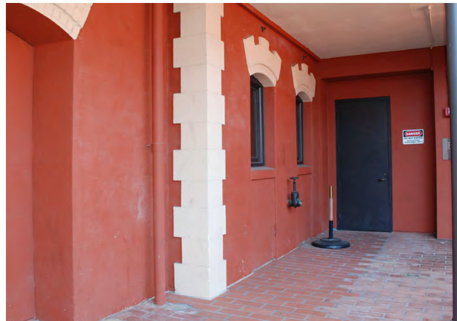
Inappropriate - some of the original Ghirardelli Buildings have areas where the original brick was refinished with cement plaster and painted to match the brick paving.
