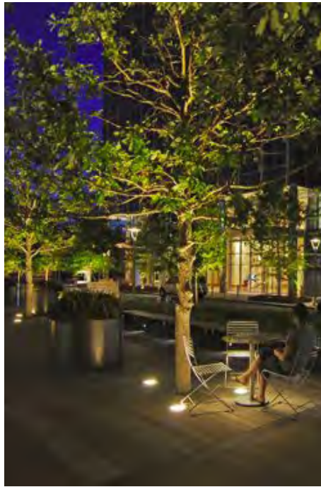
Example of appropriate tree uplighting.
