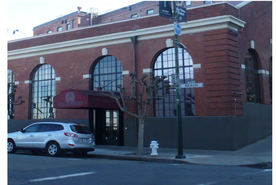
Canopy at the Power House, Beach Street facade is not appropriate in scale or shape
