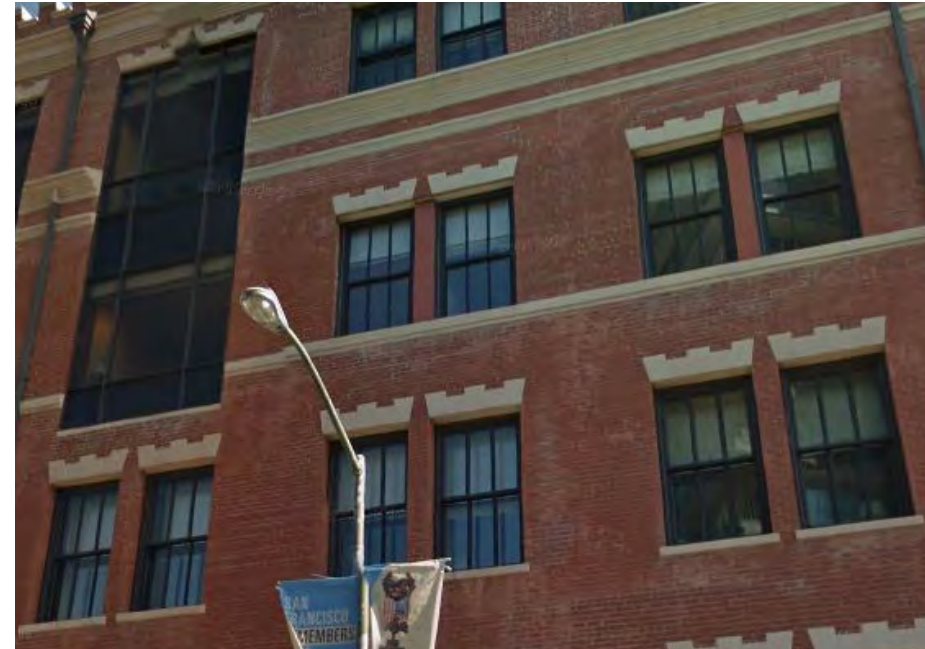
Appropriate Replacement: The double-wide windows at the Chocolate Building were replaced with new aluminum windows that closely resemble the original steel windows.
