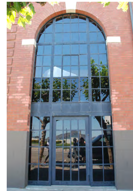
Power House: This door appears to be original and is a good example an industrial style door
