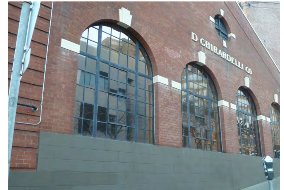
Power House: Original, industrial, multi-lite windows have been modified but retain the original character
