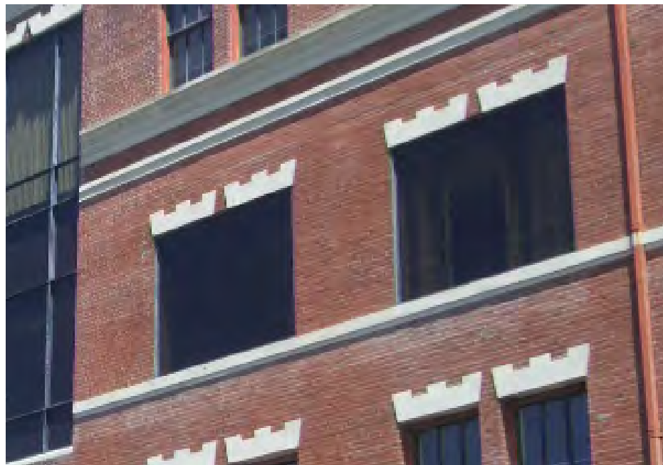
Chocolate Building: Two pairs of windows were replaced in the 1960s with fixed metal windows that spanned two openings
