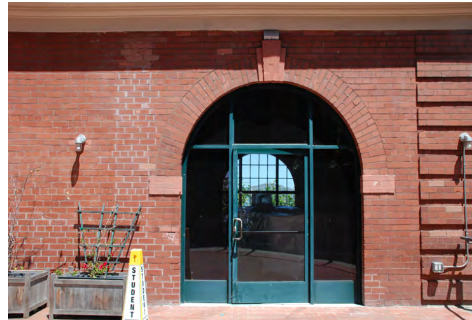
The style of the door/storefront system is appropriate. However, a darker color such as bronze or black would be more in keeping with the Power House's industrial character.
