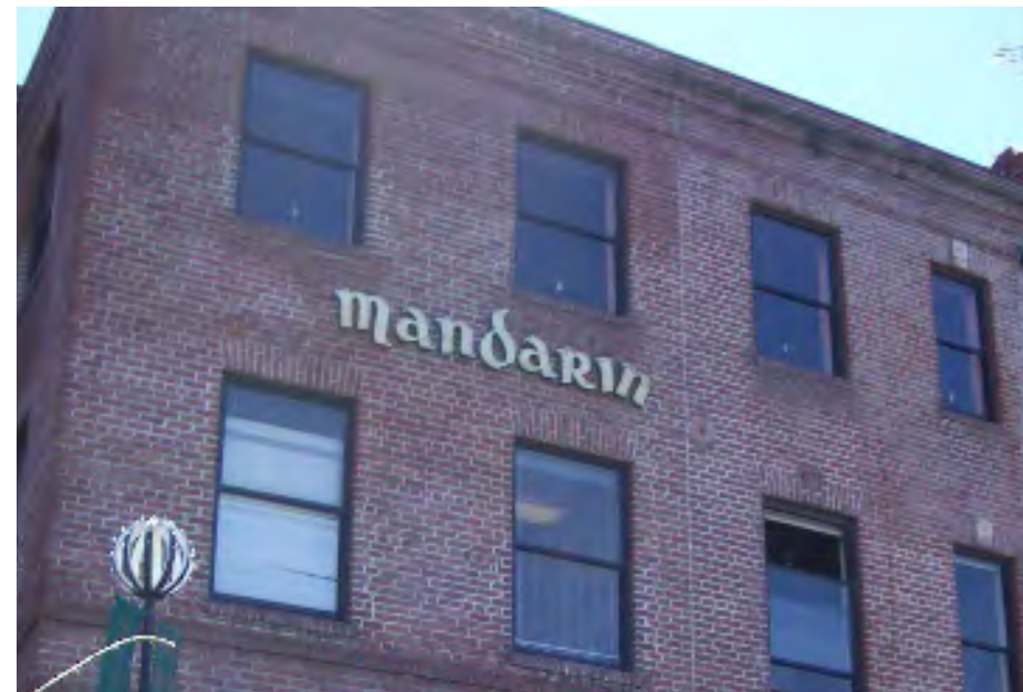
Appropriate Replacement: Original windows were replaced with aluminum windows that have a contemporary look. Though distinct from the original, they continue to give the facade a uniform look.
