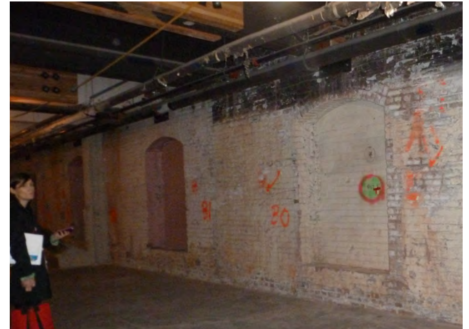
Interior view of windows at basement level of Cocoa Building that were filled in
