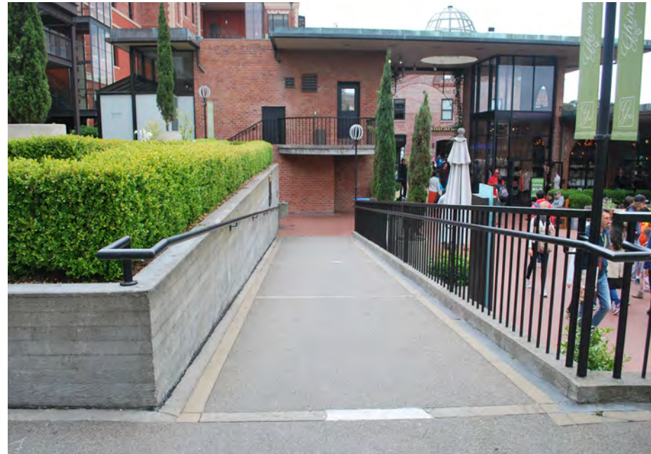
Some existing slopes do not meet ADA standards.
