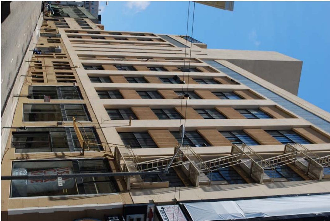
Top photo: Double-hung wood sash window typical of those in the second through fifth stories. The sash dates to 1916, while the corrugated sheet metal spandrels must date to 1947-1948.
