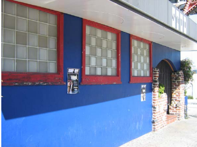
Detail of entry on Harrison Street, south façade. Source: Page and Turnbull
