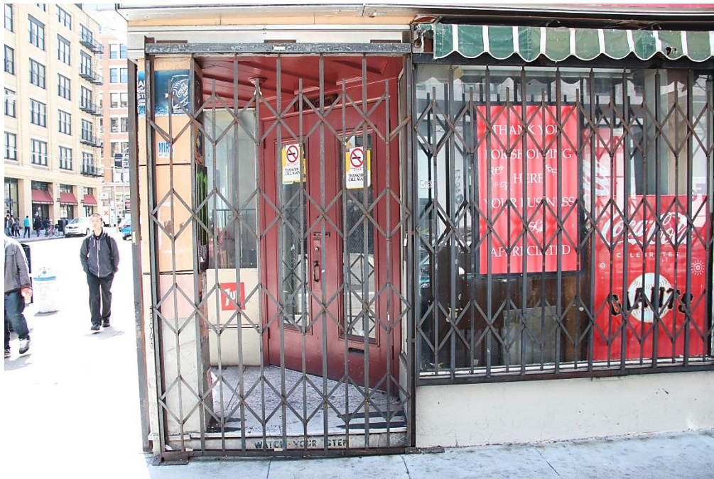
Corner storefront addressed as 600 Mission Street. Note mosaic tile threshold and paneled ceiling.
