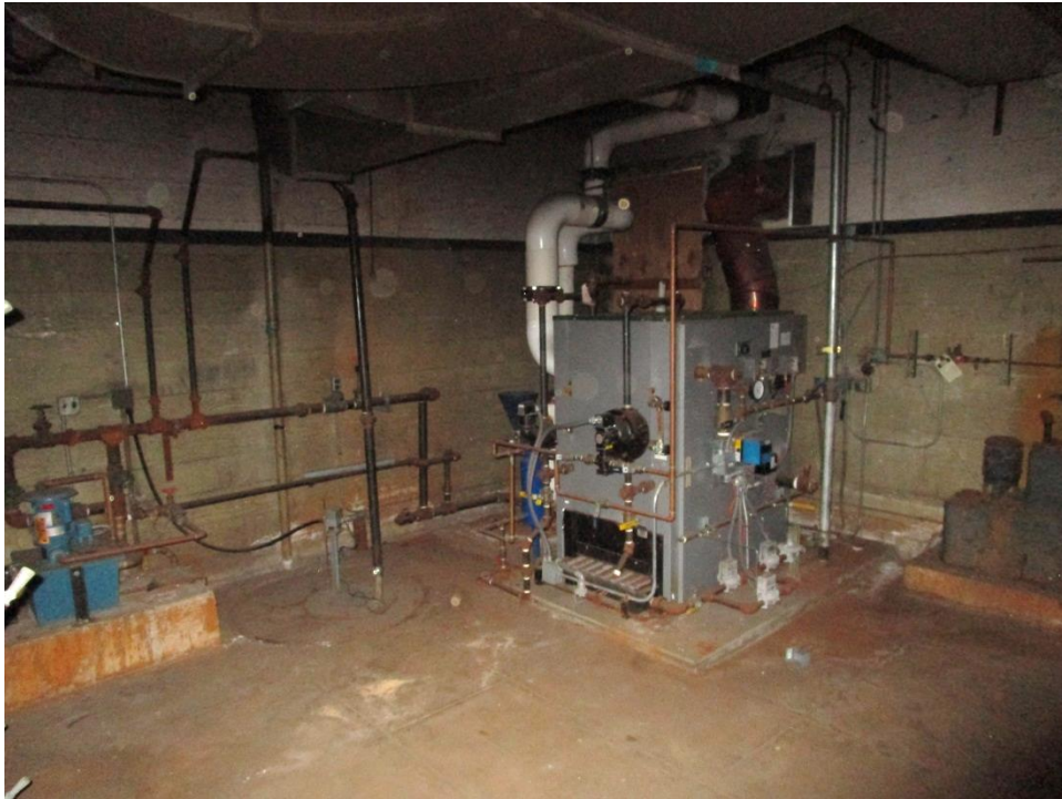
Basement boiler room showing apparent connection to 45 Onondaga Avenue
