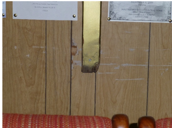
Figure 16: Ends of gold crucifix have missing paint. Wood paneling has abrasion marks from furniture.
