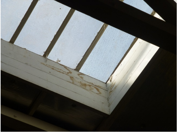
Figure 21: Water damage to wood paneling near skylight.
