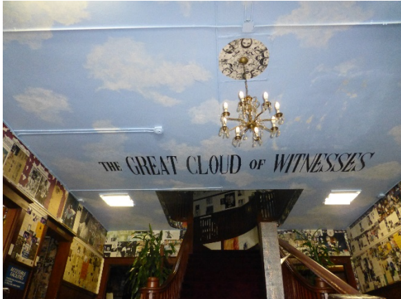
Figure 7: Painted ceiling appears to be in good condition with no flaking or chipping paint.
