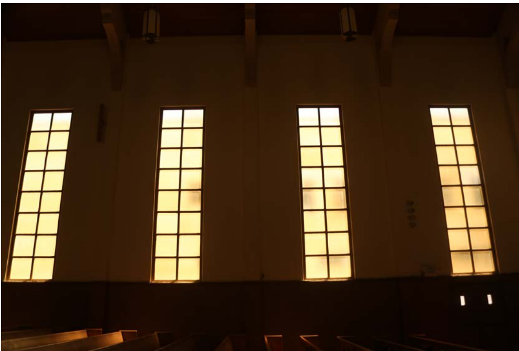
Vertical wood sash ribbon windows with divided lites and yellow glass, east interior wall.
