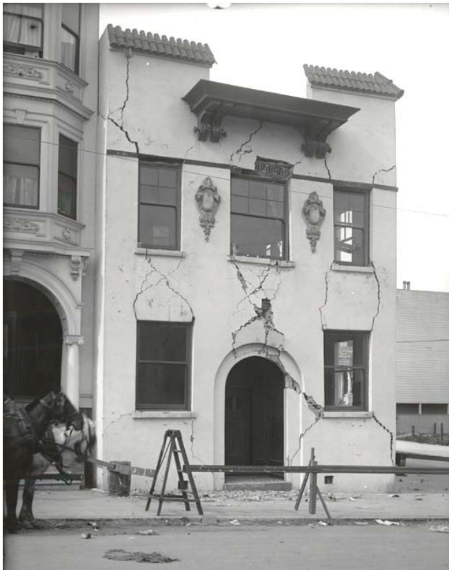
1950-1952 15 th Street, designed by August Nordin and constructed in 1901 as a can factory for Edwin Bennett. This brick masonry building was heavily damaged during the 1906 Earthquake and subsequently replaced. (Bancroft Library)
