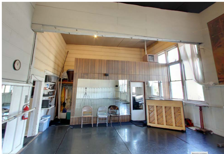
View west within Lodge Room No. 2. Note the Howe Truss has been enclosed with boards. (Google Maps)
