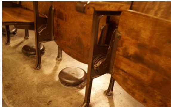
Figure 41. Heating units beneath seats.
