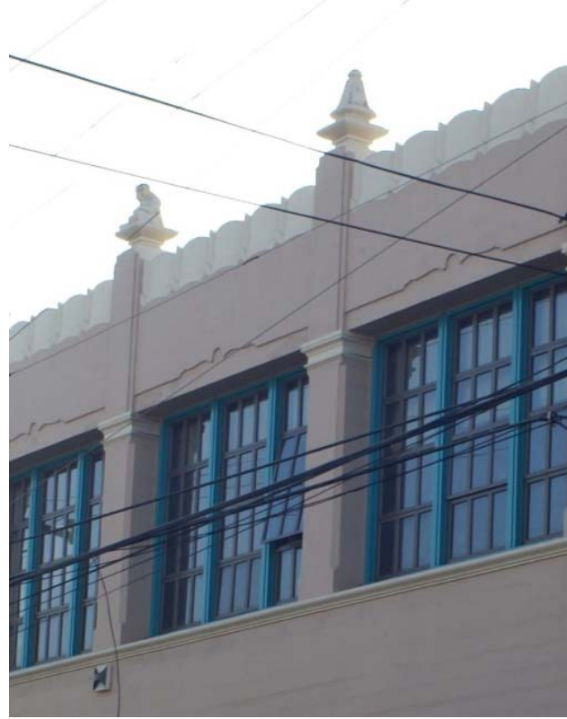
Figure 19. Typical condition at second floor level of east classroom wing facing Bryant Street.
