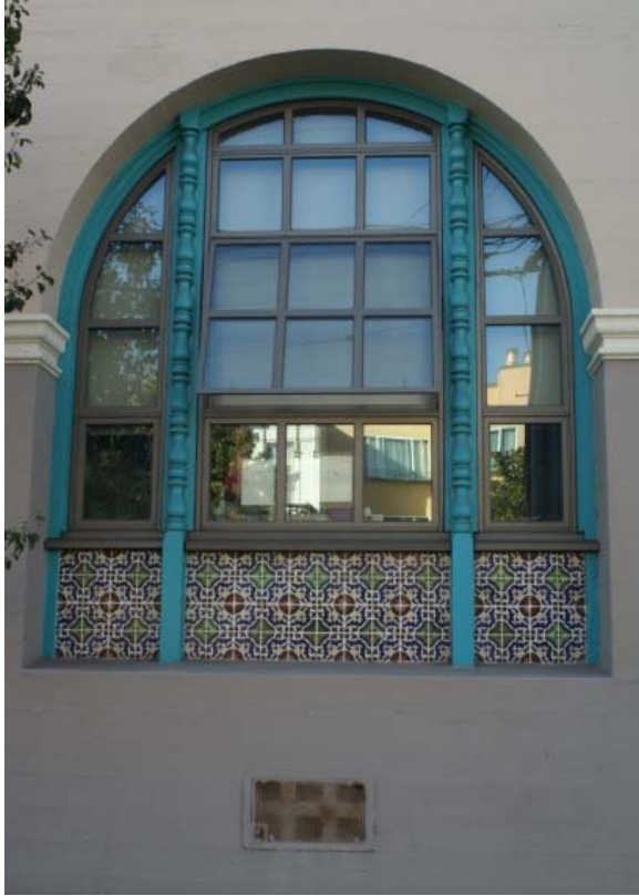
Figure 18. Typical window on first floor level of east classroom wing facing Bryant Street.
