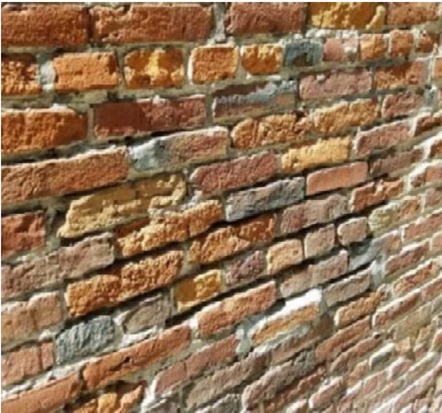
Close-up showing variations in brick and mortar, 2017. Source: Page & Turnbull, Inc. (2017) report
