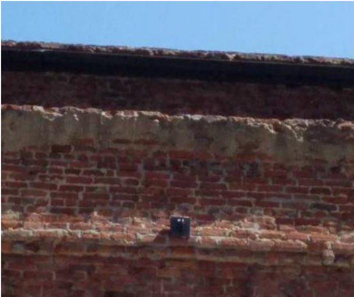
Close up of patched bricks at cornice, 2017. Source: Page & Turnbull, Inc. (2017) report
